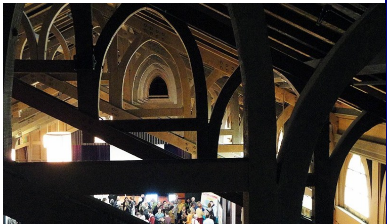
Wood trusses punctuating clerestory lighting at Merrill Hall are exposed rather than concealed, resulting in better indoor air quality. Photo: Alan D'Souza.
