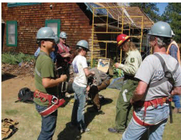
OHP Historian Amanda Blosser (second from left) with fellow volunteers preparing to replace the roof of the 99 year-old Cedar Lodge near Susanville
