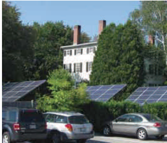
A solar panel installation that is not recommended
