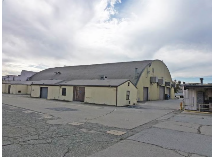
Image 2. View looking south at the northwest and northeast façades of Hangar 4 and Building M.
