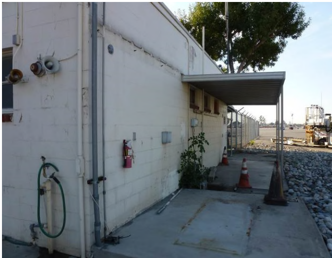
Image 7. Detail view looking west at the north façade of the personnel quarters.
