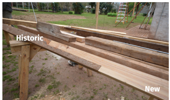
This historic cypress rafter has a new cypress piece sistered in to replace damaged material. The darker wood is the historic material that was retained. Image Credit: NPS|Sarah Marie Jackson.
