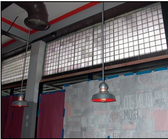
Original leaded-glass transoms were rediscovered and preserved during the Blaze Pizza rehabilitation project.
