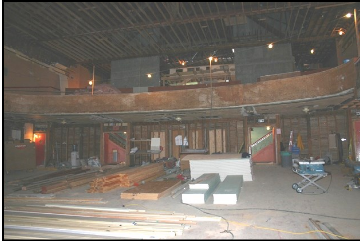
Main auditorium during restoration. Among the challenges was removing a destructive colony of bats.
